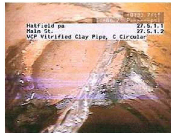
GROUND WATER IN SANITARY SEWER SYSTEM
