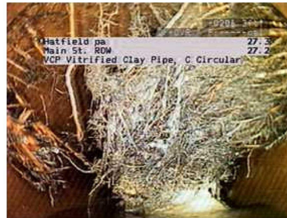
ROOTS IN SANITARY SEWER SYSTEM
