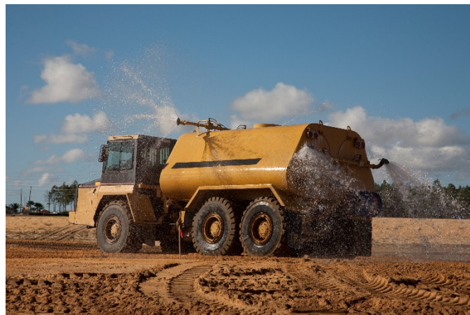
A truck equipped with a spray system can spray water throughout a construction site and prevent dust from being transported off-site.
